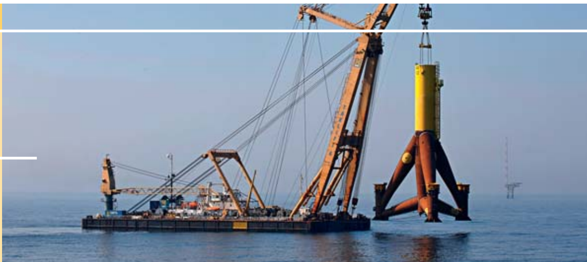
Fig. 2 A floating crane transports a tripod structure for an Areva Wind turbine into the construction field. Photo: AREVA Multibrid / Offshore foundation / Jan Oelker
