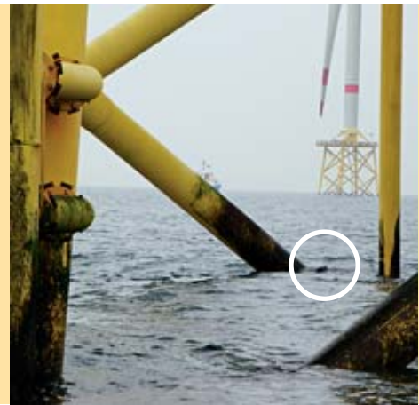
Fig. 27 Seal on a wind turbine foundation in spring 2011 Photo: BSH
