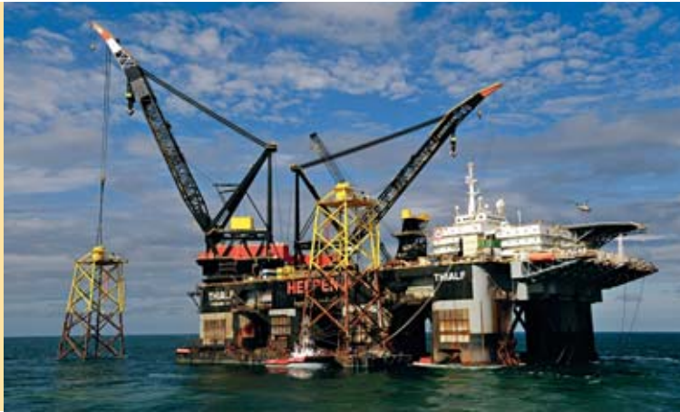
Fig. 6 The large THIALF offshore work platform lifts a jacket foundation into position. Photo: DOTI 2009
